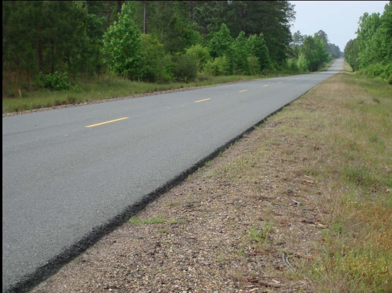
LA 464 (Vernon Parish) – 2001 with “Plain” RAP Shoulders TYPICAL SHOULDER DROP-OFF
